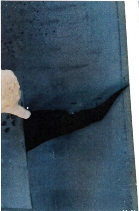
1' tear in membrane along flow path of water.
