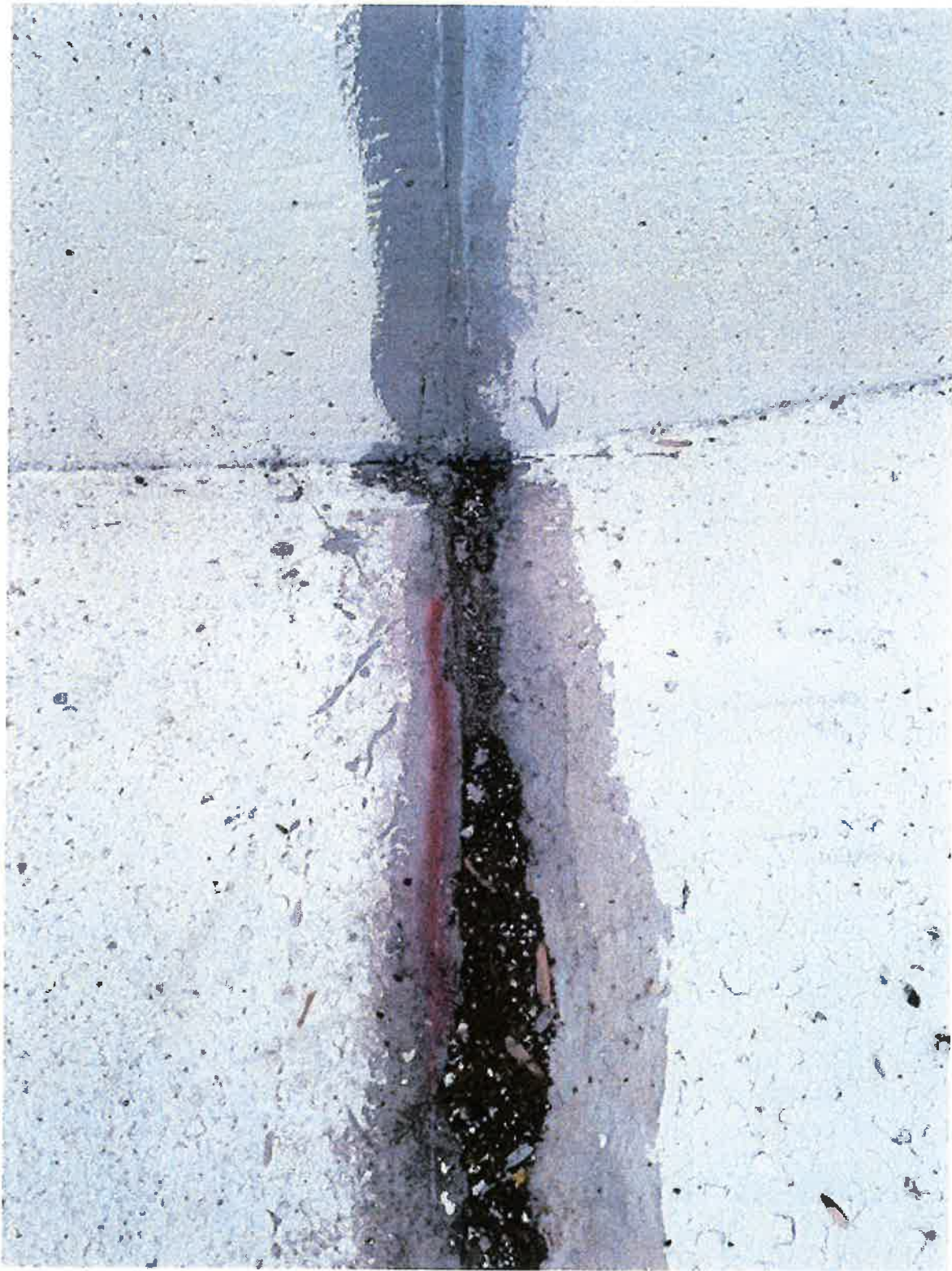
Figure 5 LEAKING BRITTLE CONST. JOINT
