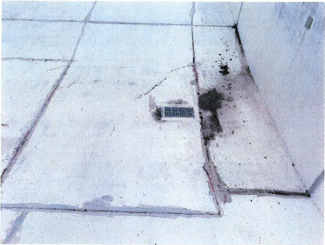
Figure 4 CONCRETE STRUCTURAL CRACK
