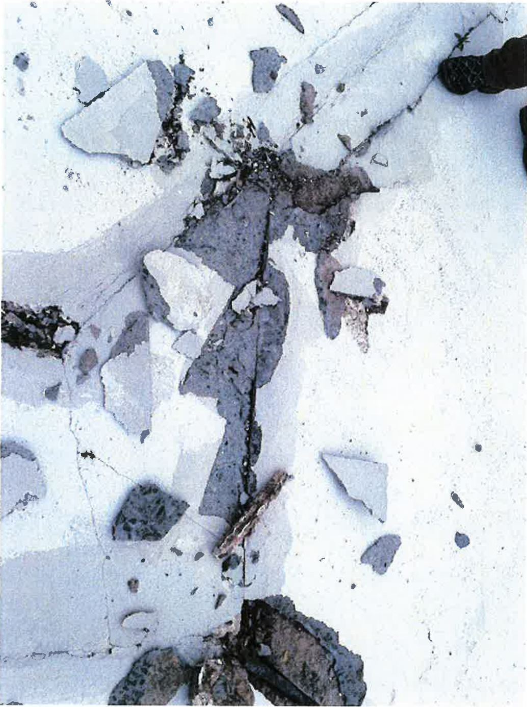
Figure 3 CLOSE UP OF WEATHERED JOINT
