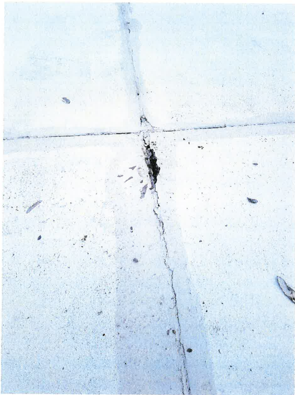
Figure 7 JOINT WITH DETACHED CONCRETE SEAM
