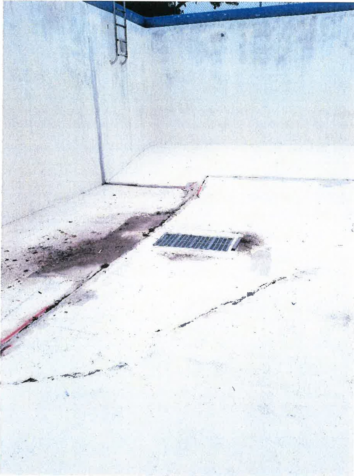
Figure 6 DEEP END POOL WATER LEAKAGE
