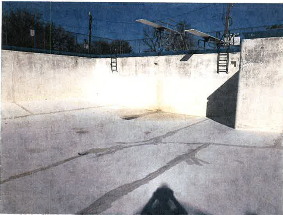
Cracks in deep end floor.
