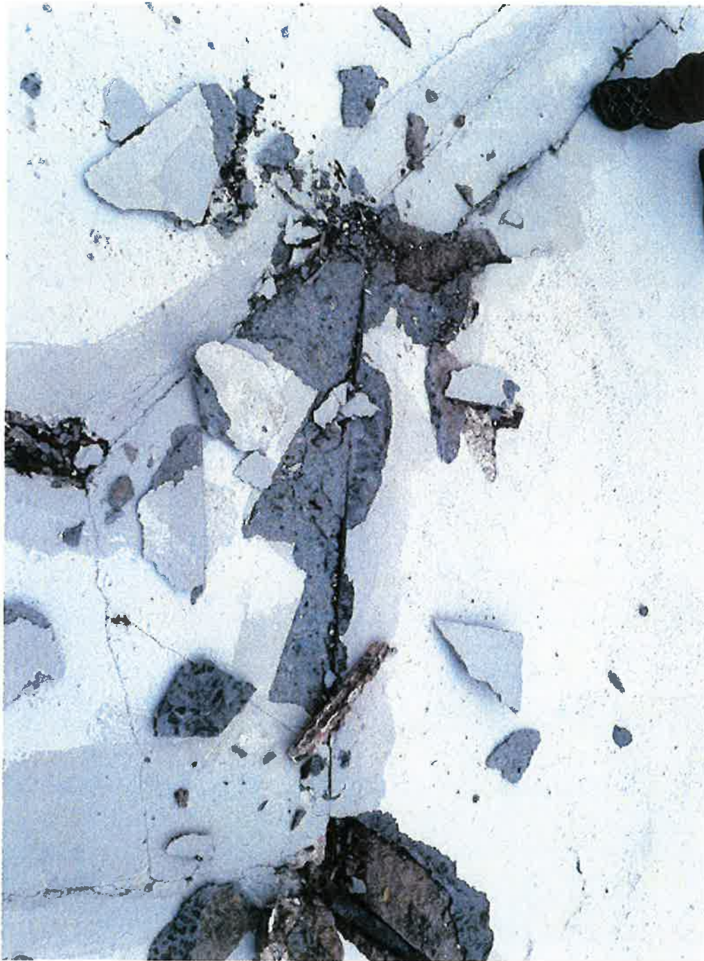
Figure 3 CLOSE UP OF WEATHERED JOINT
