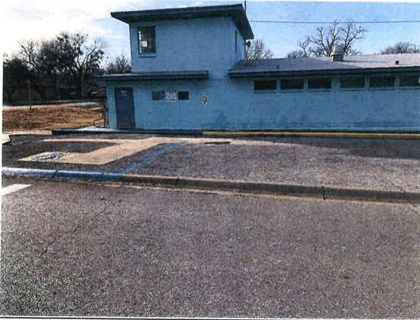
Parking, entrances, counters are not in A.D.A. compliance
