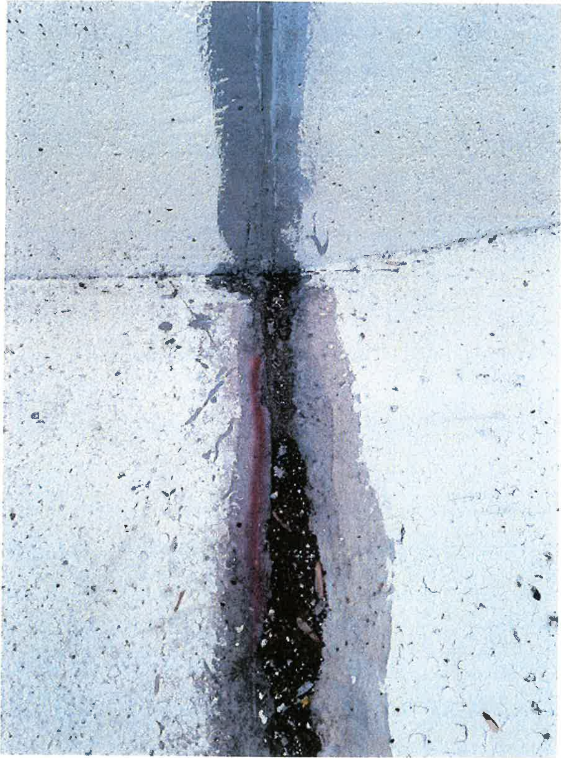
Figure 5 LEAKING BRITTLE CONST. JOINT
