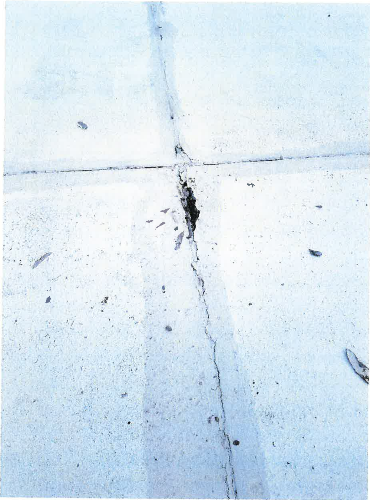
Figure 7 JOINT WITH DETACHED CONCRETE SEAM
