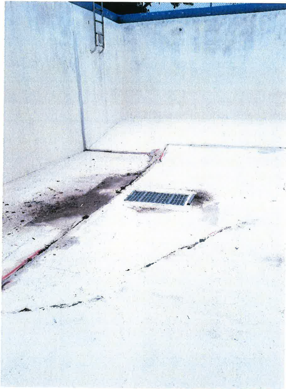
Figure 6 DEEP END POOL WATER LEAKAGE
