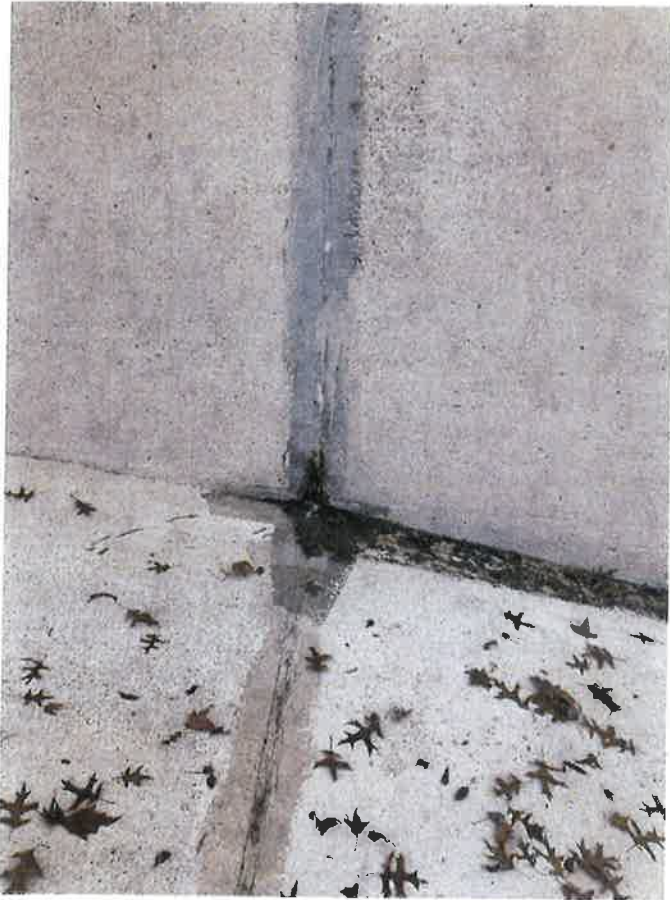
Crack leaching water.
