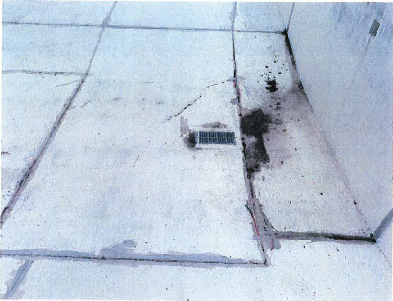
Figure 4 CONCRETE STRUCTURAL CRACK
