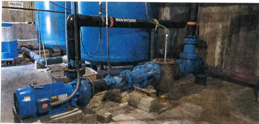
Pump motor, strainer, filter, chlorinator
