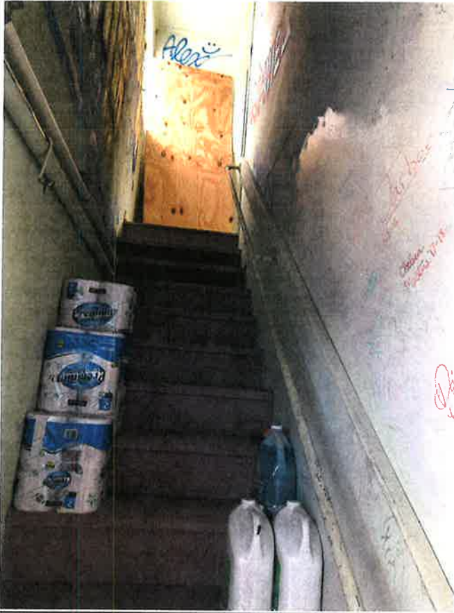
Abandoned upstairs in bathhouse.
