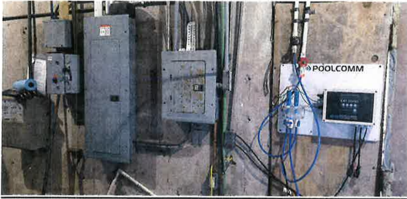
Electrical and Pool Controller.
